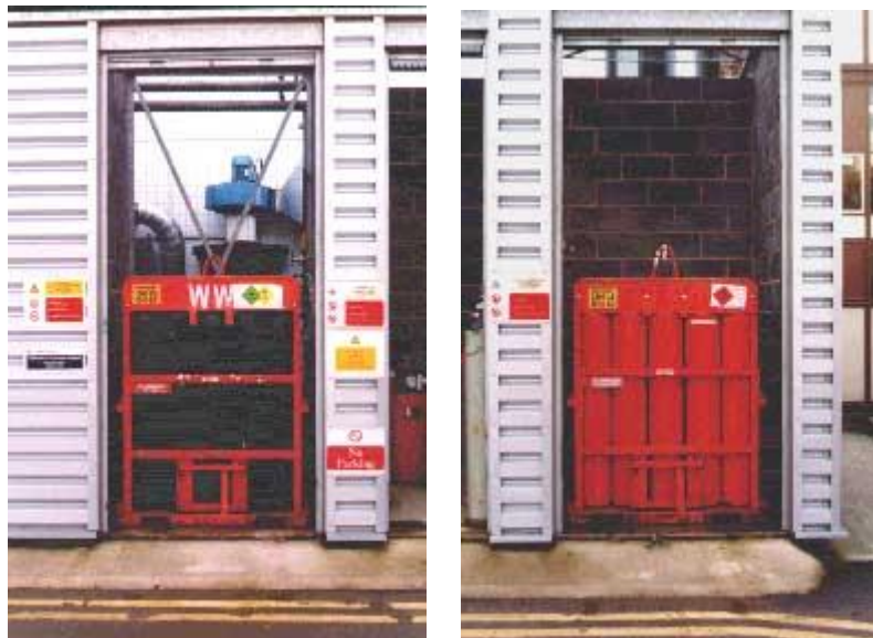
Figure 6: Purpose built stores for oxygen and hydrogen (Pictures courtesy BOC gases)
